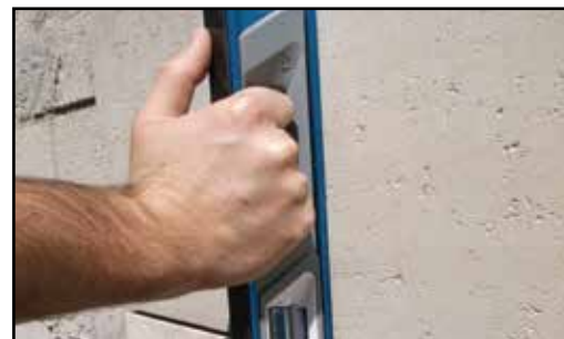
Use a large level to check and maintain an even-face plane over multiple tiles.
