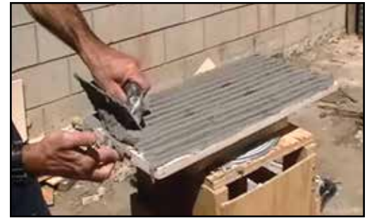
Use a 1/2" notched trowel to apply non-sag polymer-modified thinset bonding mortar to the back of the stone.
