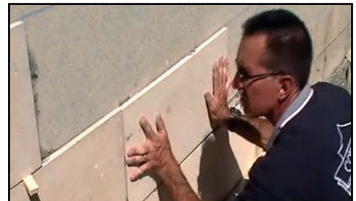
Work the stone into the wall using a left-to-right motion until the mortar squeezes from the perimeter of the tile and full-coverage adhesion is achieved.
