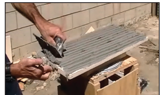
Use a 1/2" notched trowel to apply non-sag polymer-modified mortar to the back of the stone.
